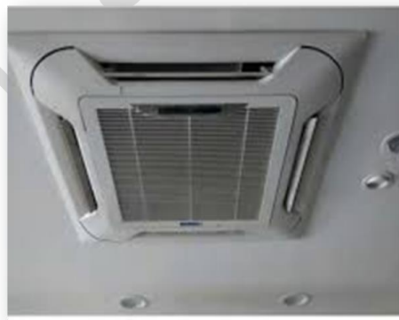
Centralized Air-Conditioning System
